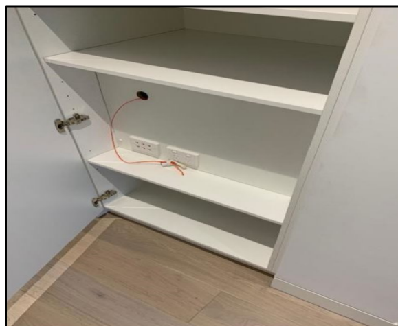
Figure 15. Typical built out shelf
